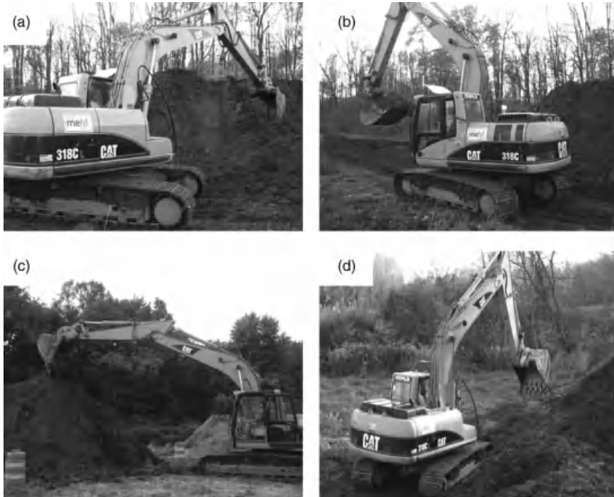
Figure 8.81 The work cycle used in this test lasted about 1 min. (a) Take a full scoop; (b) Rotate 90–180° and travel 30 m (100 ft); (c) Dump load and rotate 90–180°; (d) Empty return of 30 m and start with next cycle.
