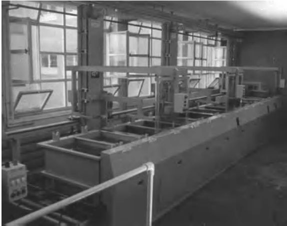
Figure 6.70 Fully automated electroplating unit for rack parts or barrel goods with continuous bath analysis and treatment steps, such as filtration. Illustration courtesy of Carl Dittmann GmbH & Co KG.
